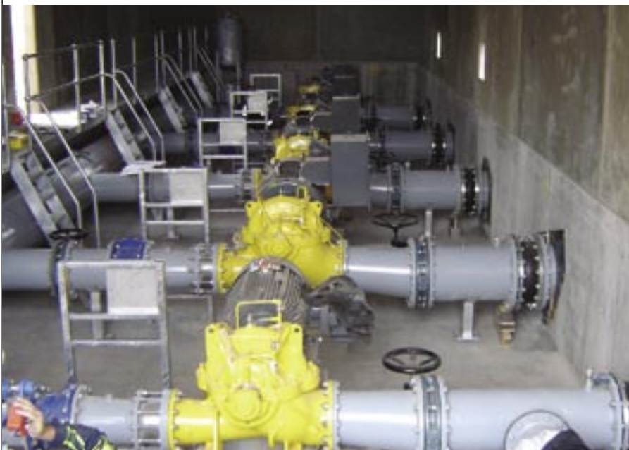
A View of the new pump station
