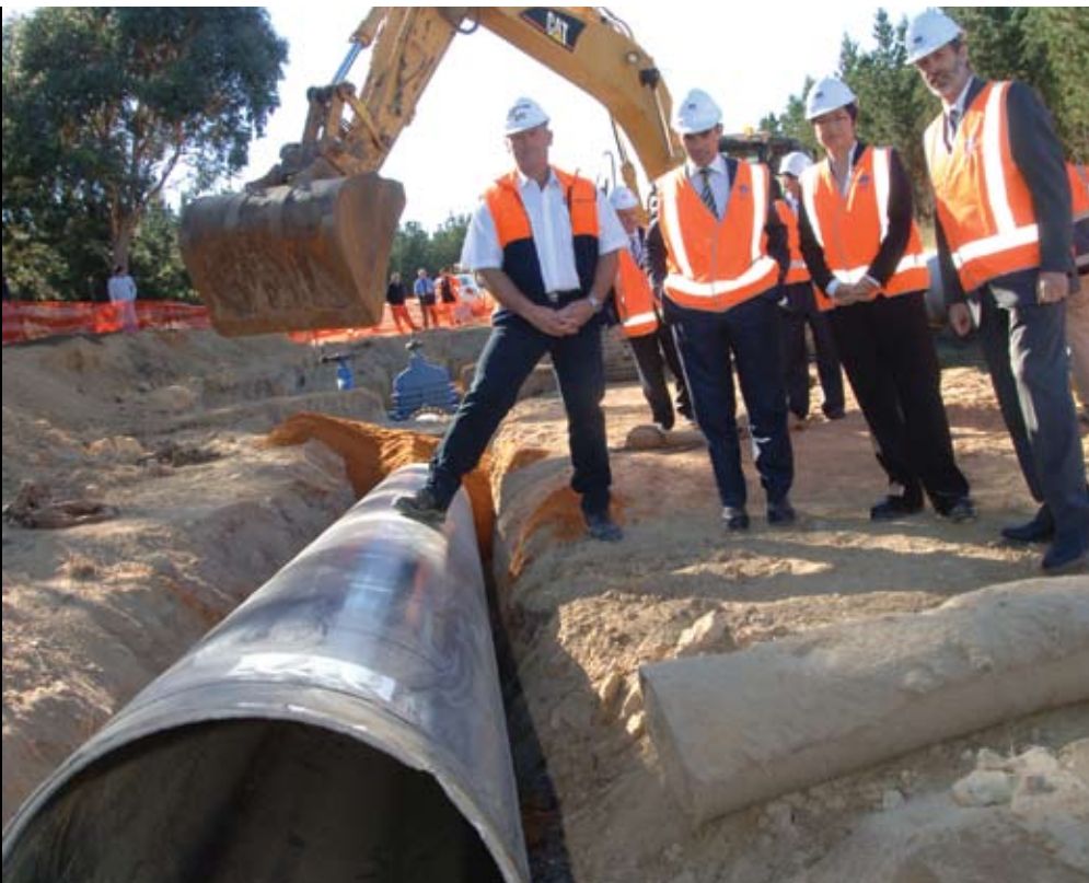
Connecting the final section of Superpipe are, from left, Pipecon Managing Director Andrew Mahar, State Water Minister, the Hon. Tim Holding, Federal Minister for Climate Change and Water The Hon. Senator Penny Wong and Central Highlands Water Chairman John Barnes.
